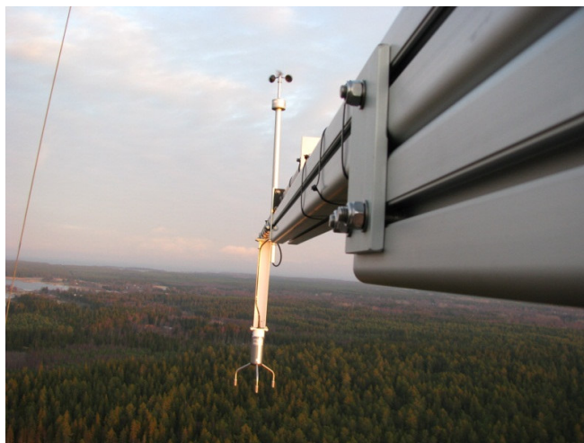
Figure 5. Installation of a mechanical anemometer Vaisala WAA151 and an ultrasonic anemometer Vaisala WS425 to same measurement boom at Site A. Other sites applied the WMT702 ultrasonic wind sensor.
